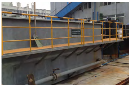
Air Flotation Tank
