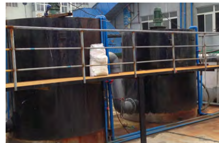
No. 2 pH Adjusting Tank/ Reaction Tank
