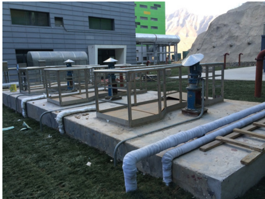
Reaction tanks and concentration tank (underground)
